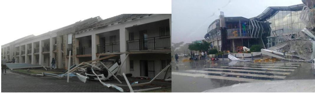
Figure 1: (left) An apartment complex in Fourways significantly damaged by the storm. Picture courtesy of Tiro Molokele, (right) portion of the Cradlestone Mall that collapsed. Picture courtesy of Twitter @capvma
